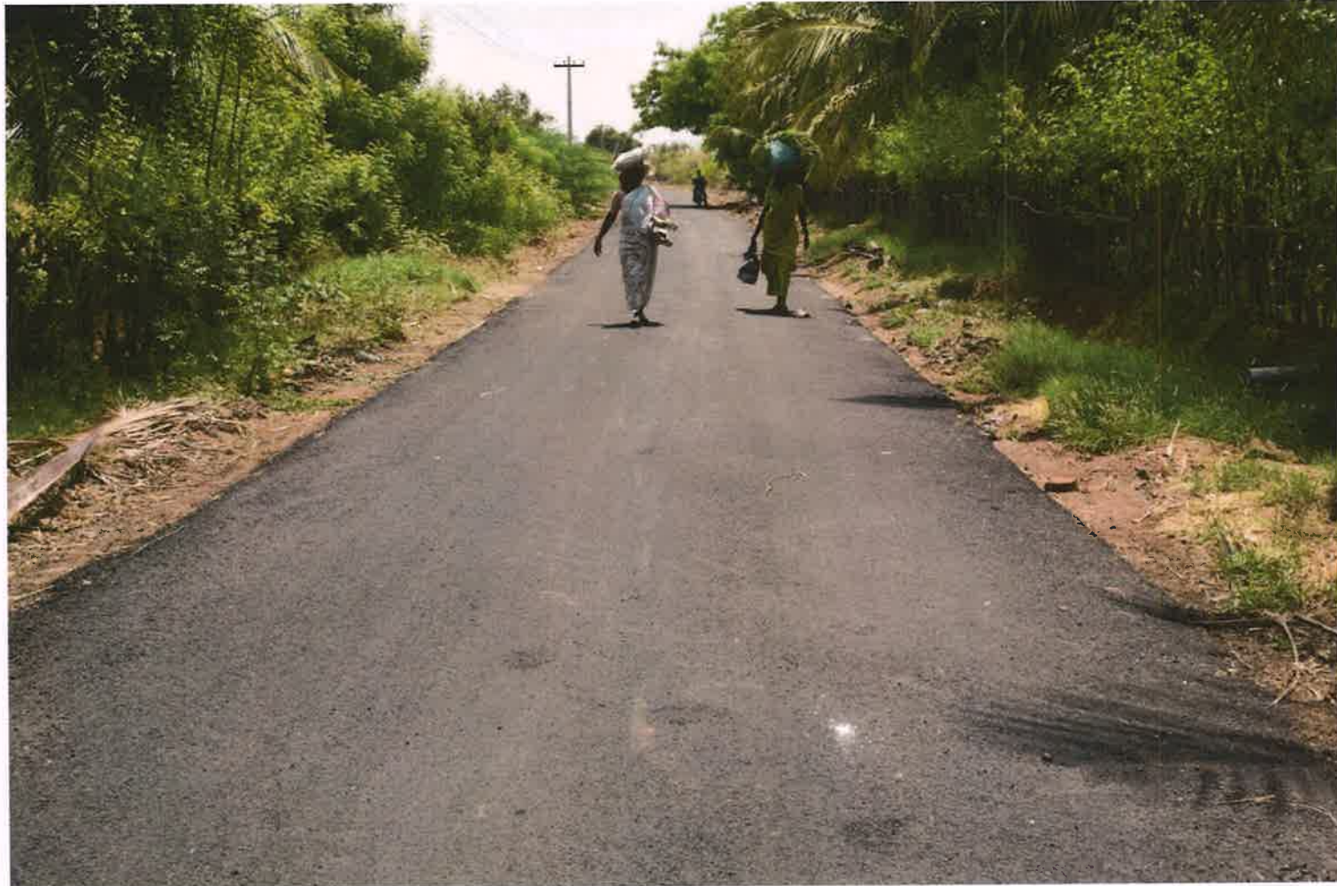
View of Black Topped road repaired and relayed by TNPL at Punjai Thottakurchi village
