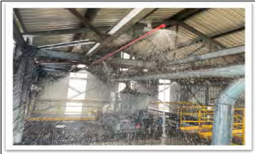
Water sprinkling system at coal storage yard
