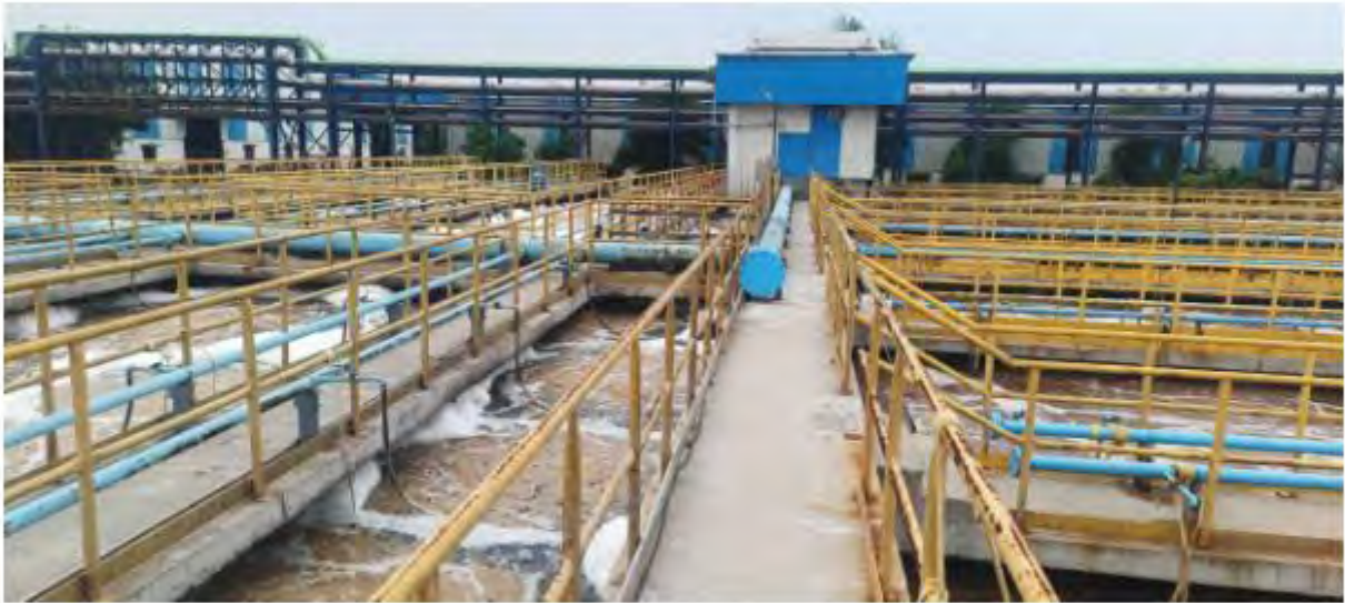
MOVING BED BIOFILM REACTOR (MBBR)
