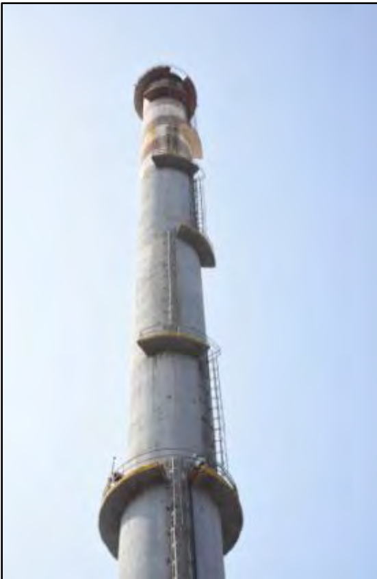
Power Boiler Stack of height 100 m
