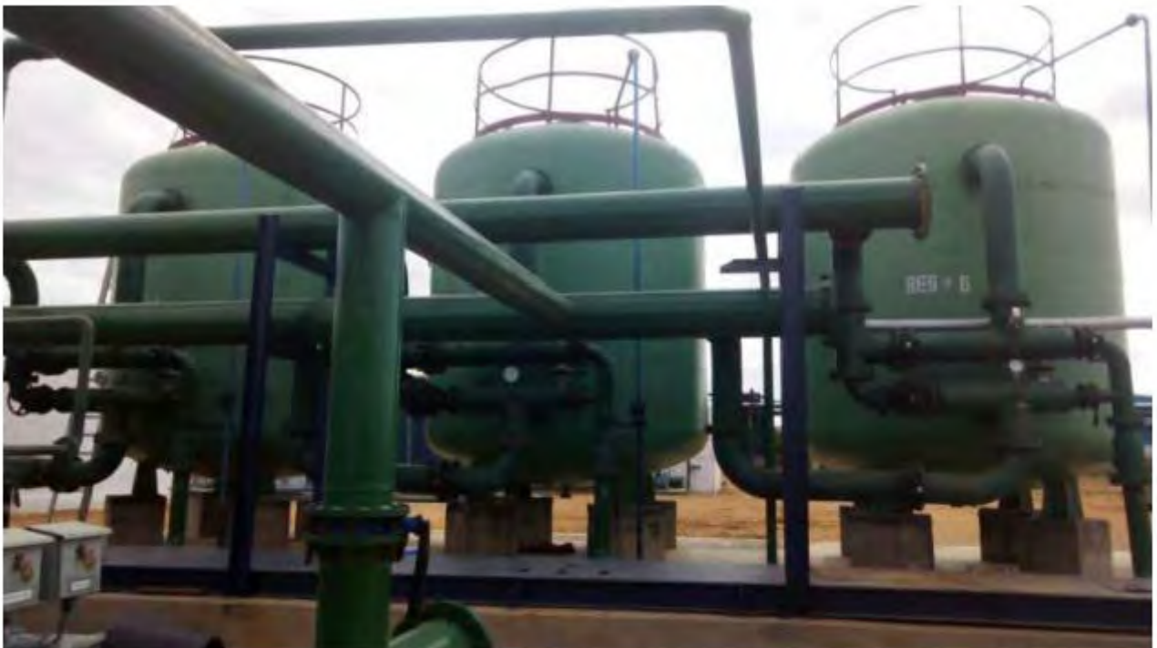
PRESSURE SAND FILTERS
