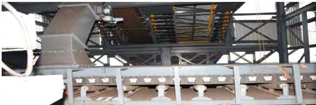
Closed transfer of coal between conveyors
