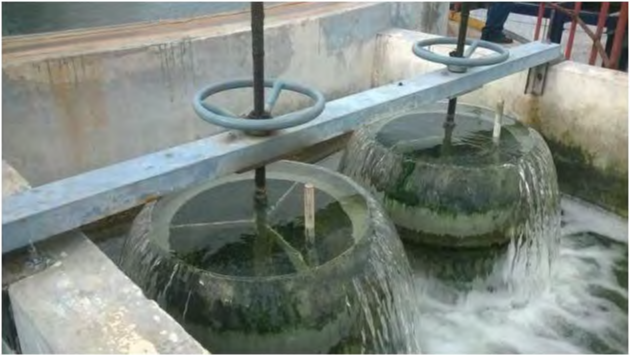
OUTLET OF DAF SYSTEM
