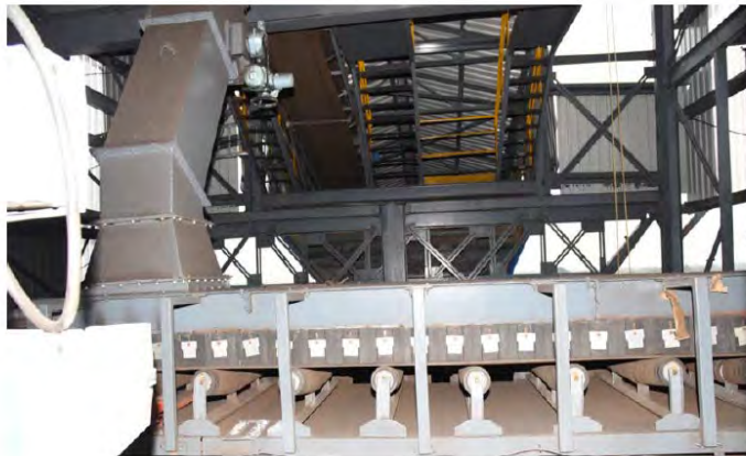
Closed transfer of coal between conveyors
