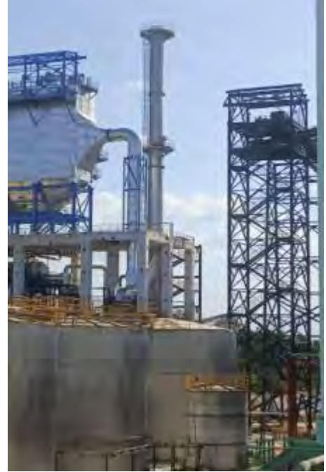
Lime Kiln Stack – 54.8 m height
