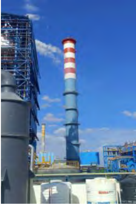
Chemical Recovery Boiler Stack – 90 m height
