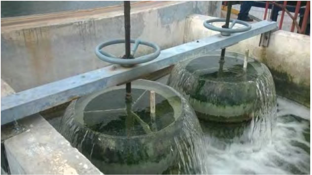
OUTLET OF DAF SYSTEM
