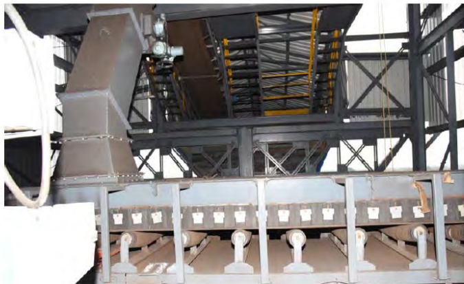
Closed transfer of coal between conveyors
