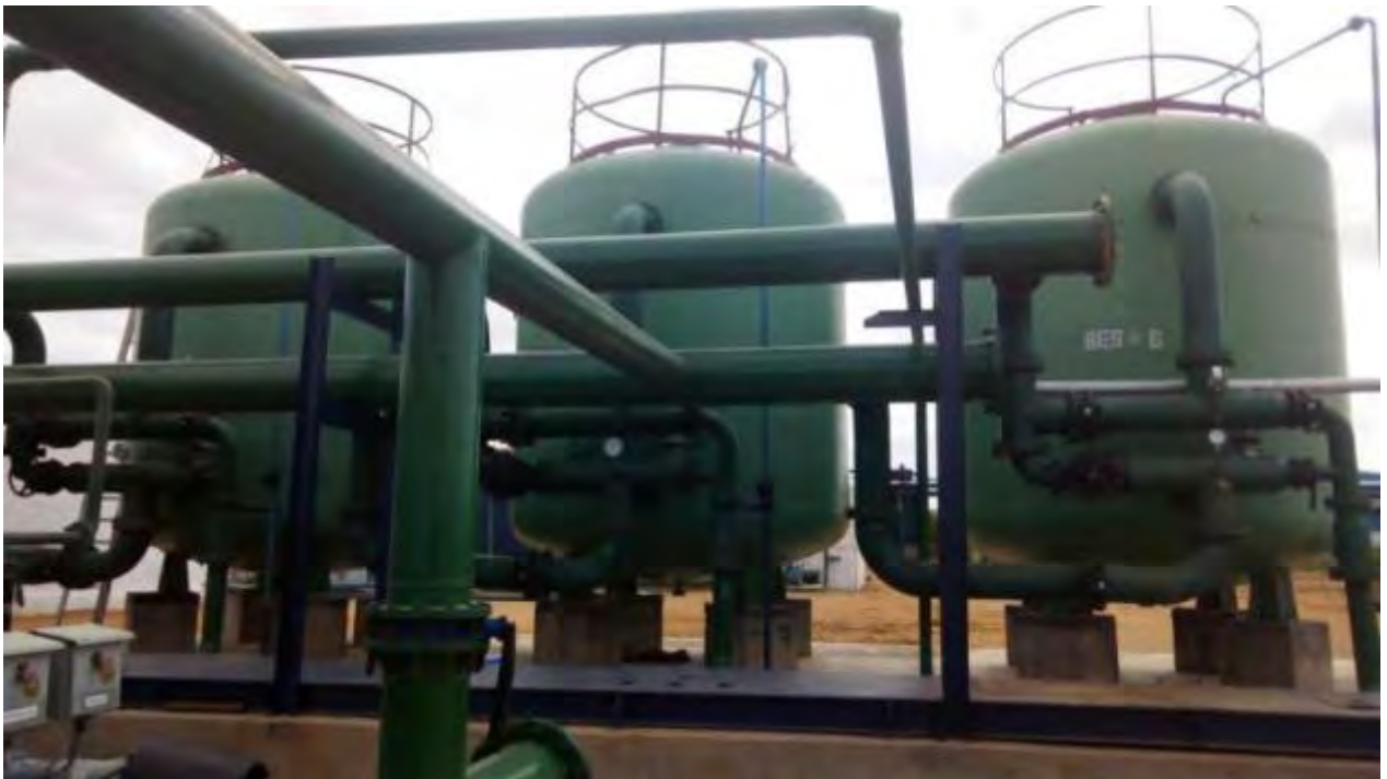
PRESSURE SAND FILTERS
