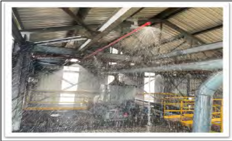
Water sprinkling system at coal storage yard
