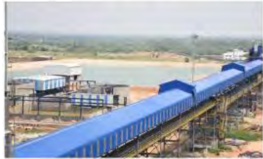
Closed hoods for coal conveyors
