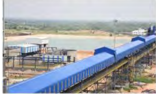
Closed hoods for coal conveyors
